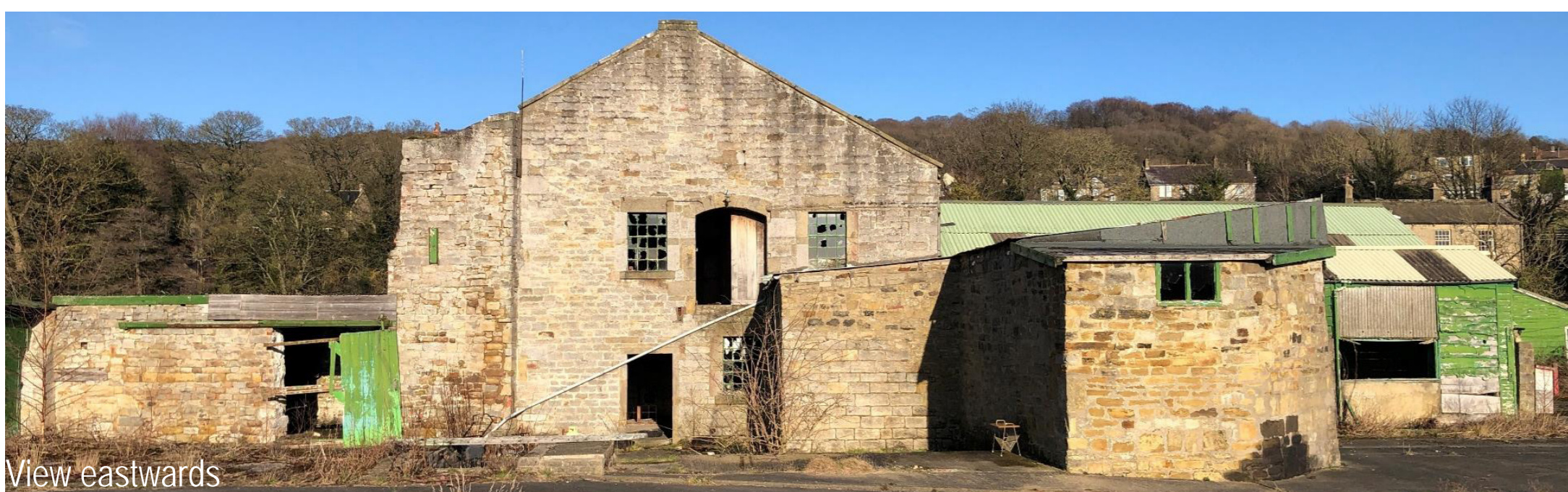
View north-west with the ancillary buildings in front of the two-storey mill
